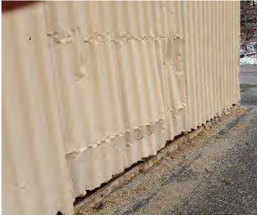
Buildings have exceeded their useful life
