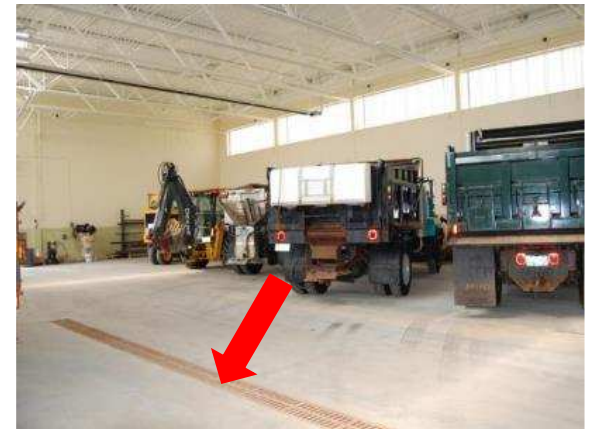
Any drips or spills from vehicles stored inside will be collected in a closed floor drain system preventing them from reaching the environment
