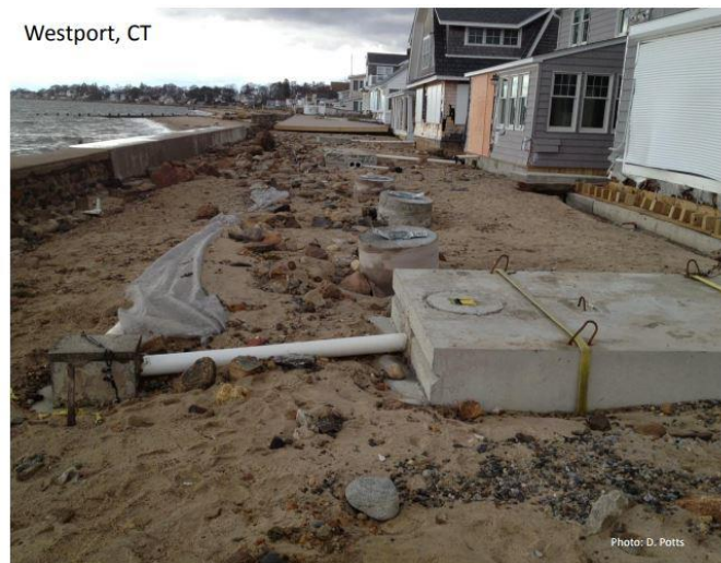
Figure 23 Exposed septic system after coastal storm in Westport, CT.
